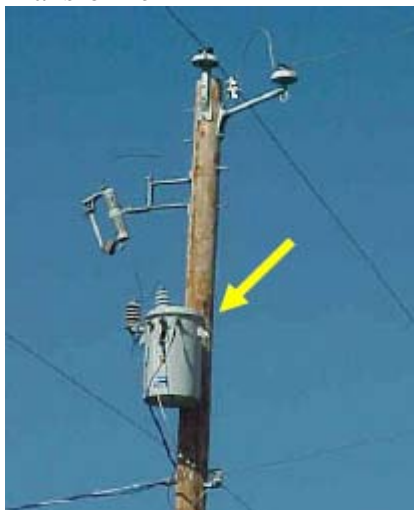
Example of a Pole-mounted Transformer
