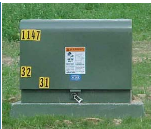
Example of a Pad-mounted Transformer
