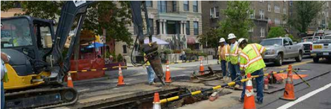
The District of Columbia Power Line Undergrounding (DC PLUG) initiative is a partnership between the District and Pepco to improve the reliability and resiliency of the Washington, D.C., electric system by placing select systems underground.
