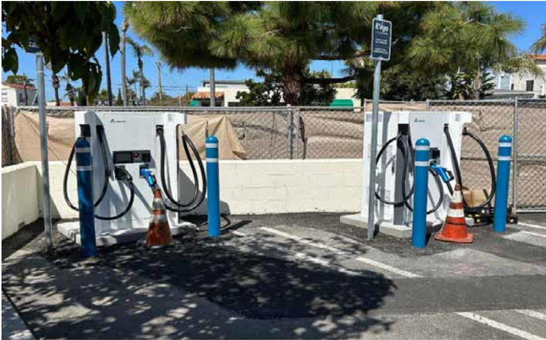
EV charging stations can offer two-way charging in the years to come, becoming a minor generational resource for a microgrid.
