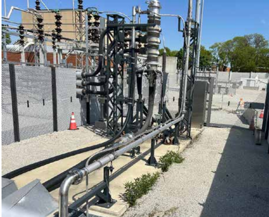
Installed in 2021, these 3000 A super conductors terminate into cables that lead to transformers on the opposite side of Northwest Substation providing a redundancy and improved reliability. Cables can be side by side because there is NO thermal heating or derating.
