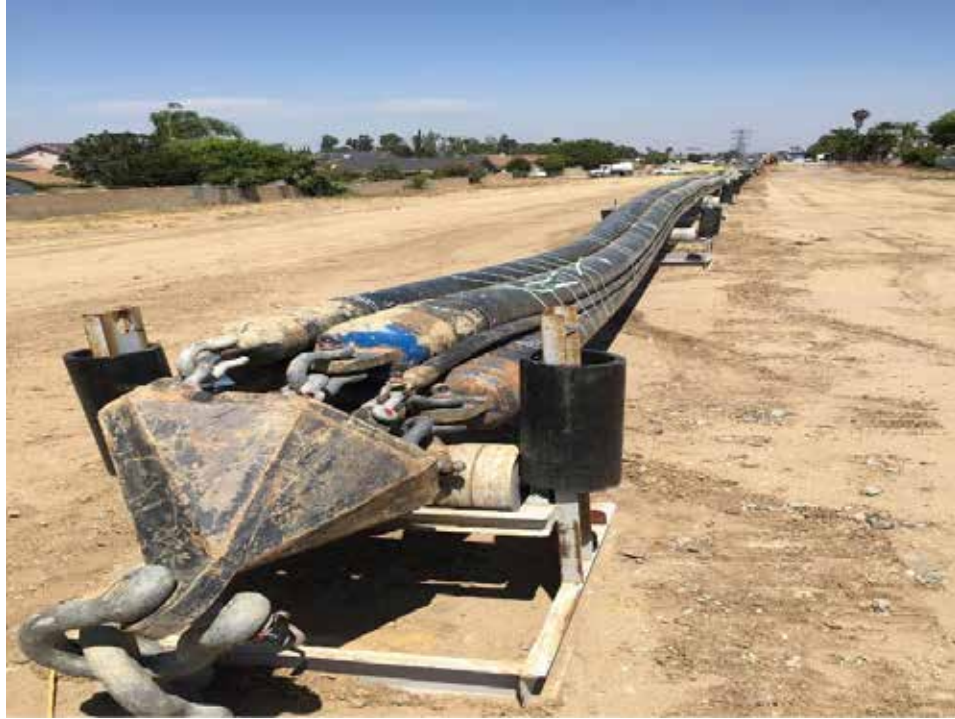
This 500kV cable at SCE should last 50-100 years if operated within design specifications.
