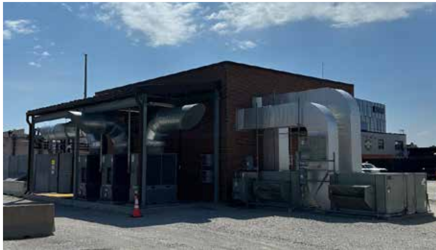
Liquid Nitrogen refrigeration for superconducting cables is a perfect insulator. This refrigeration plant at ComEd's Northwest Substation uses older technology on a closed loop system and requires regular maintenance. Newer technologies have improved dramatically.
