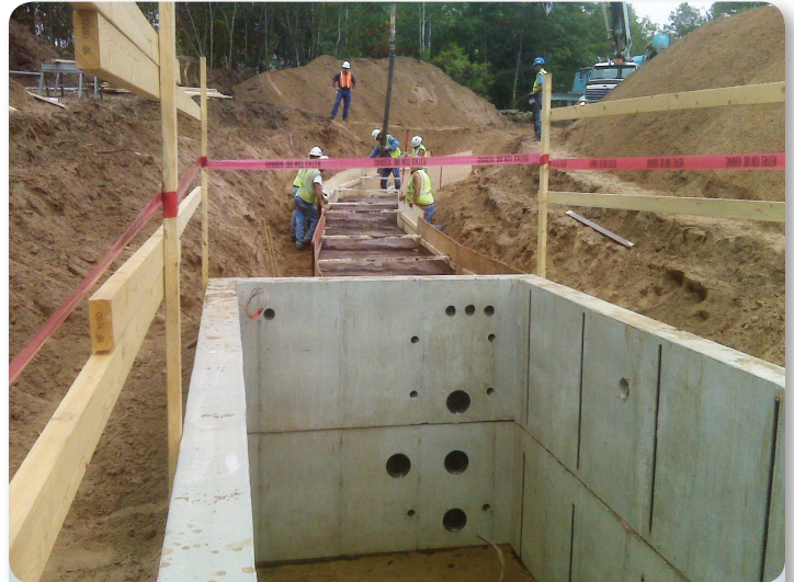
Crews work on an underground duct bank extending from a typical 8'x8'x24' vault.
