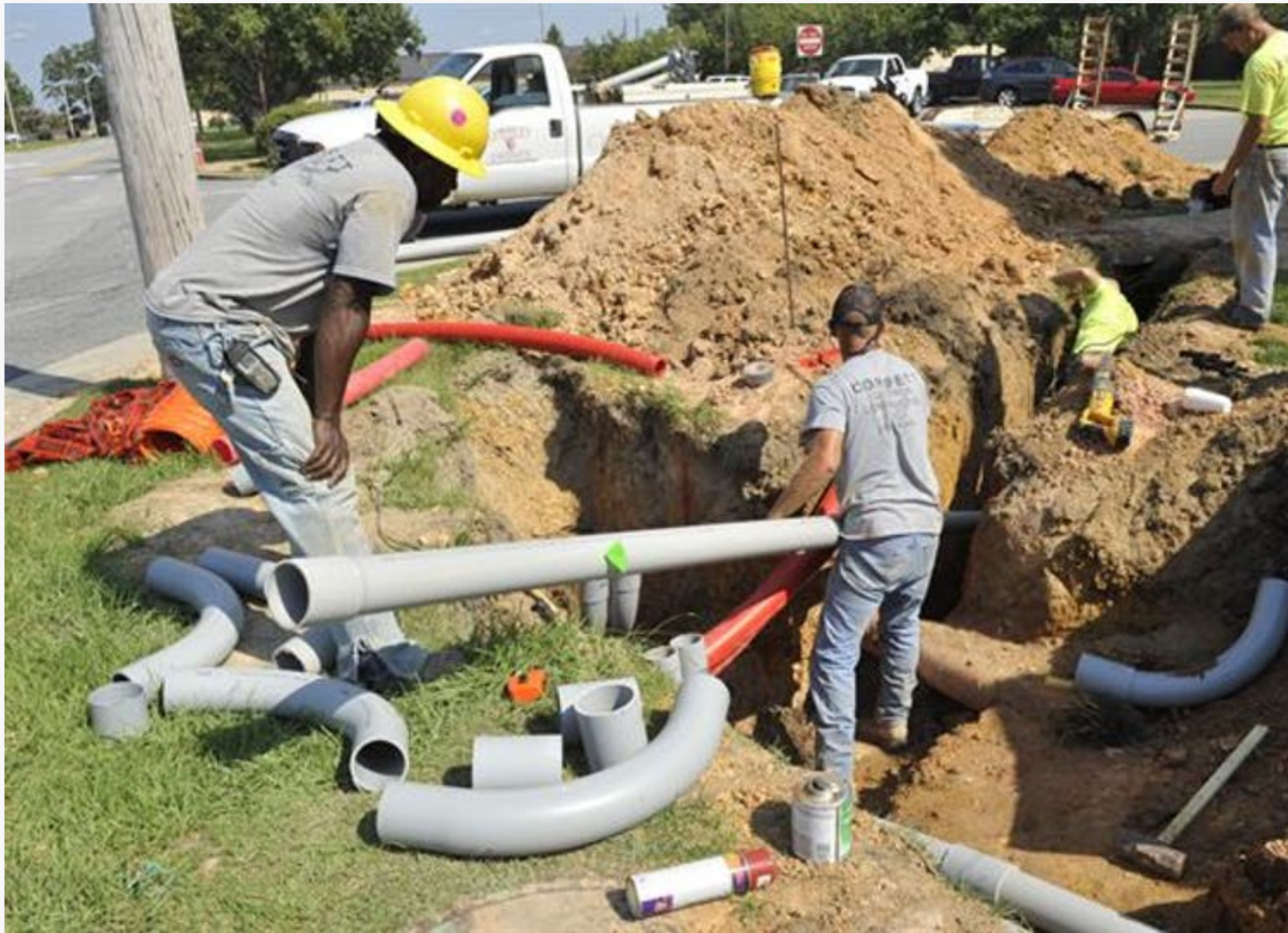
Construction at the Moody Air Force base in Georgia to put power lines underground in 2009. Image: U.S. Air Force photo by Senior Airman Schelli Jones /creative commons.
