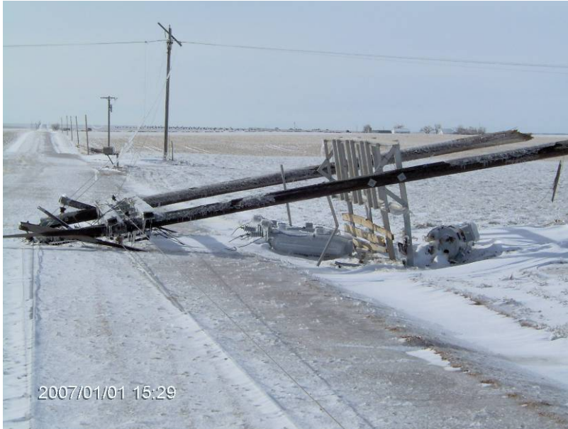
Figure 1.7: Failure of a Wooden Structure. (Source: FEMA, 2008)
