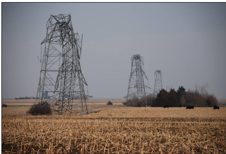
Figure 1.6: Failure of a Series of Steel Lattice Structures. (Source: FEMA, 2008)
