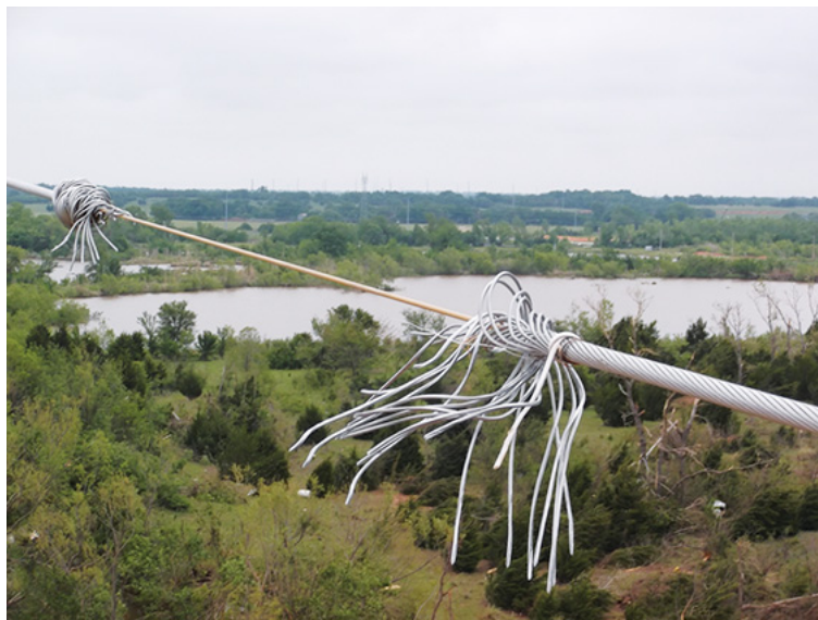
Storm damage – ACCC core remained undamaged
